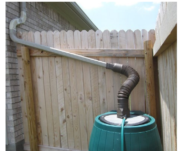
Rainwater harvesting can take the form of a greywater system (left) or a low-tech barrel in one's backyard that stores rain for a future dry day (above).
