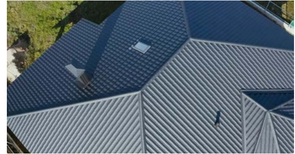
Metal roofs can be a safer decision in wildfire prone areas than other roofing materials.
