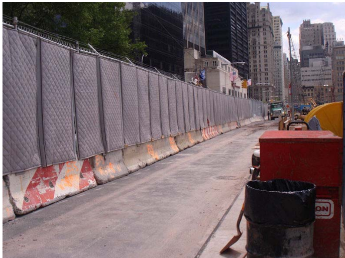
K-Rail Temporary Fence & Acoustic Material
